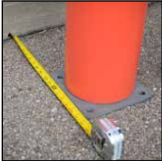
DO NOT PLACE WITHIN 10" OF ANY CURB
